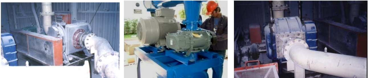
Pneumatics Conveying System
